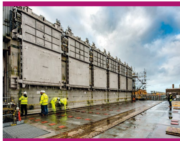
Figure 2: PFCS doors ready for retrievals
