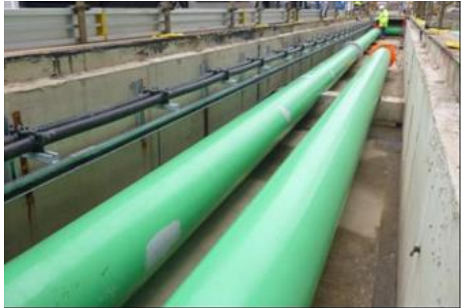
New essential cooling water pipework, reactor 22, 22B supply line
