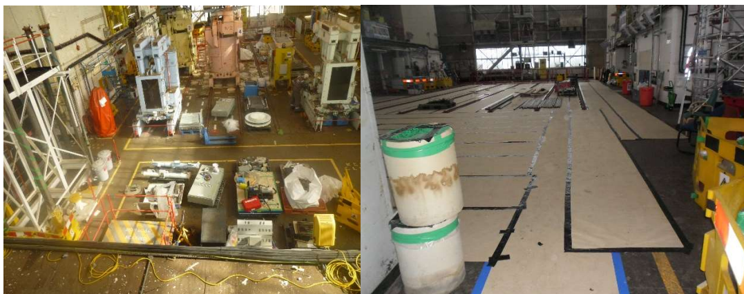
Figure 2: Before and after removal of redundant Reactor Pile Cap Fuel route equipment.
