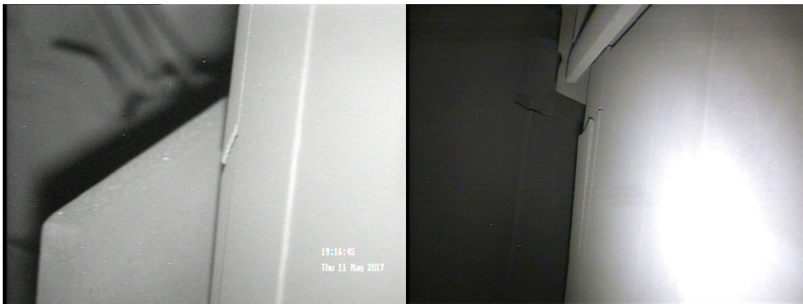
Figure 3: Left: Pronounced Crack in a Corner Peripheral Brick in TOR R1 ; found via route B51, penetration ST02. Right: Significant Branched Crack found in a Corner Peripheral Brick in TOR R2 2015
