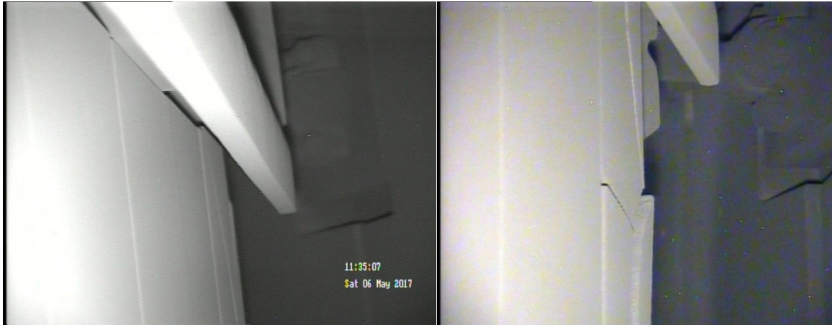
Figure 2: Left: Branched Crack in a Corner Peripheral Brick in TOR R1 ; found via route C50, penetration YZ34. Right: Significant Branched Crack found in a Corner Peripheral Brick in TOR R2 2015.
