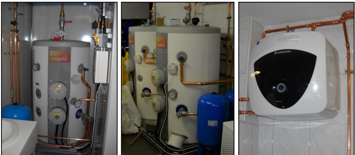
Photographs 9, 10 and 11: The newly installed “Megaflo” Calorifiers and small localised heaters
