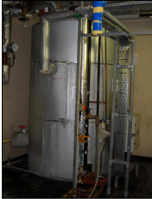
Photograph 8: One of the existing oversized and inefficient Hot Water Calorifiers
