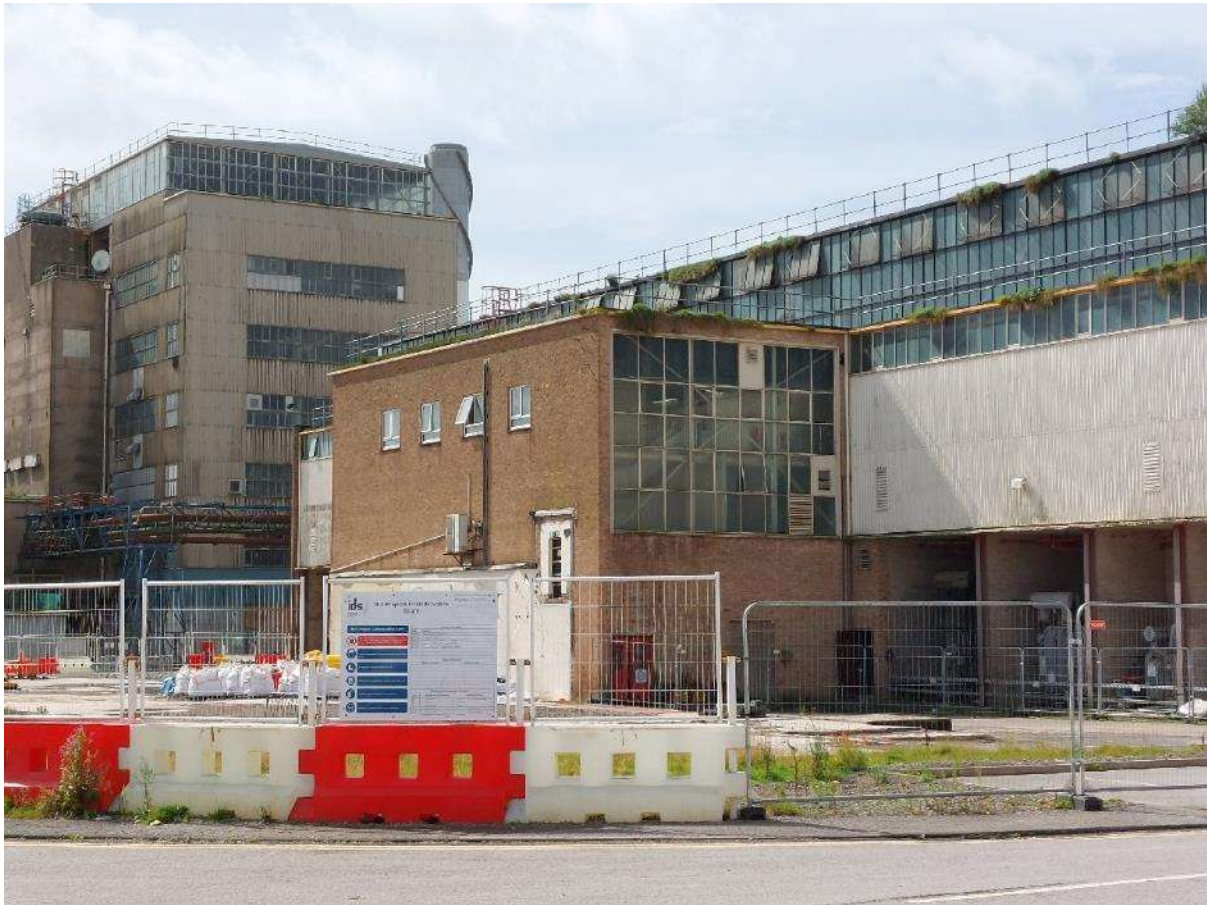
Figure 3: Turbine Hall A with in the foreground the site of the Redundant Administration Building now demolished.
